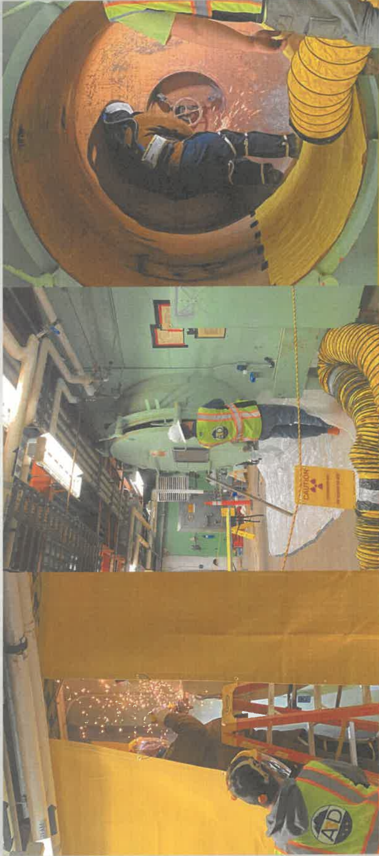
The outer and inner hatches were opened and IH monitoring occurred to ensure a safe atmosphere for the workers.
