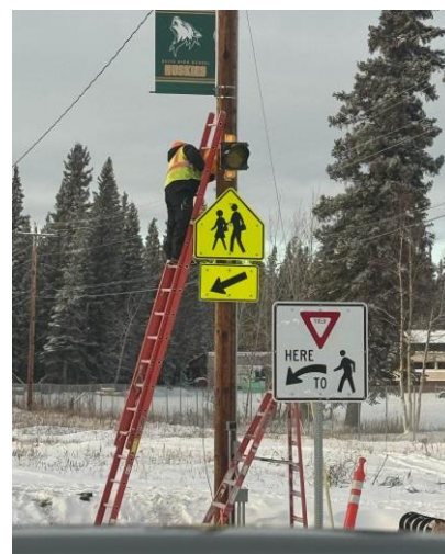
Morley Electric installed signs and lights at the school crosswalk on Nistler Road October 30, 2024
